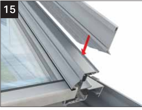
The overall length of the lean to cloaking trim is to the end of the starter bar. Cut in-line with the end of the starter bar. The tapered cut along the lower edge runs parallel with and along the gable beam top cladding.
