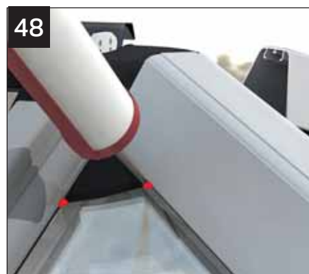
48 Discreetly 'point' the junctions between the capping gaskets and radius end flashing as shown (use new uncut nozzle).
