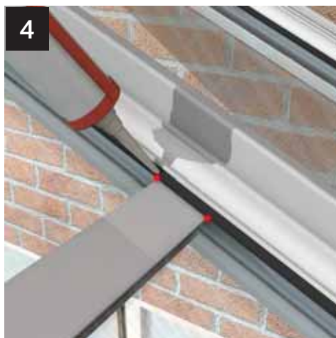
Install beads to bars. Point with appropriate sealant at the intersection between the glass jointer and bead gasket.
